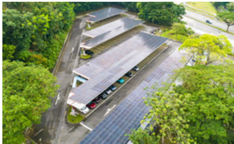
Completion of the solar-panel-fitted sheltered carpark enabled SDC to achieve and exceed its net-zero energy goal
